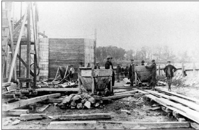
The work crew pushes cars on narrow-gauge railroad tracks to load a concrete mixer.
