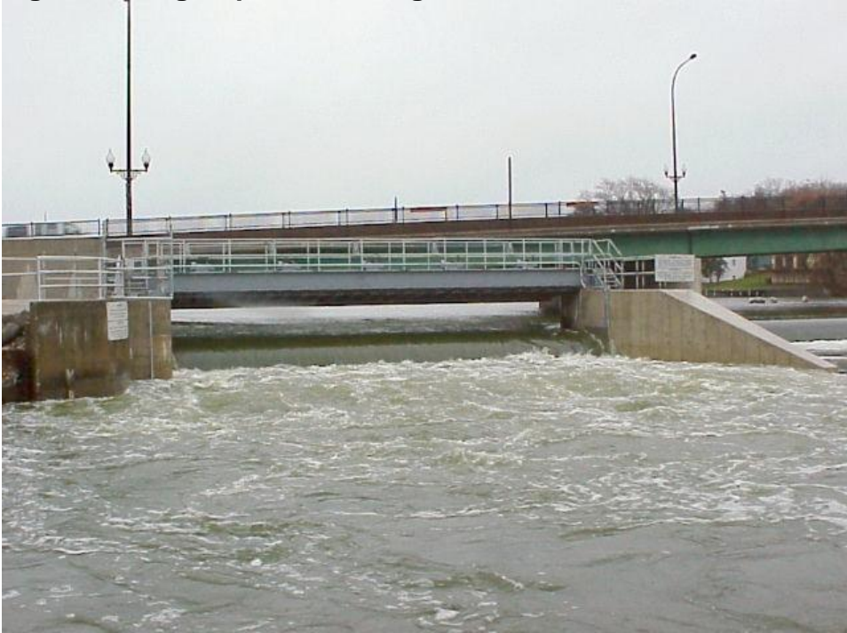
Figure 14: Algonquin Dam Hinged Crest Gate
