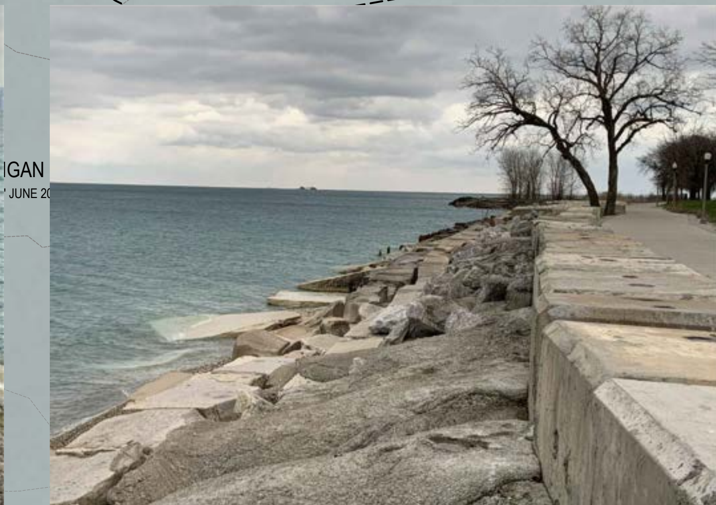
PHOTO B EXISTING DETERIORATED REVETMENT, GROUTED RIPRAP, AND LARGE CONCRETE BLOCKS
