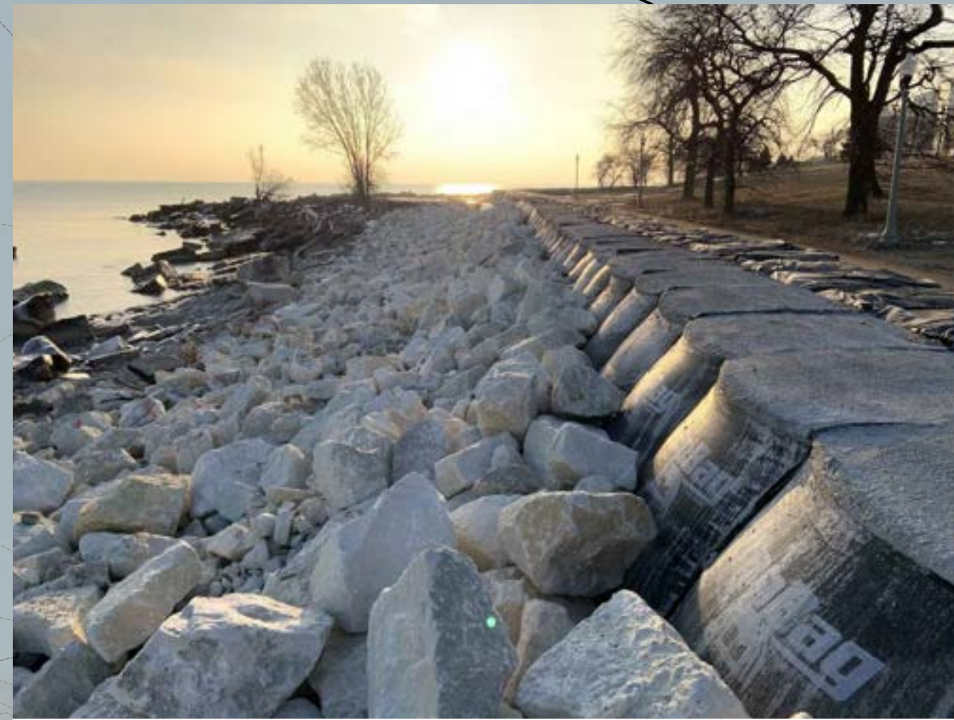
PHOTO C EXISTING RIPRAP AND CONCRETE-FILLED AND BIRD'S EYE SAND TRAPBAGS
