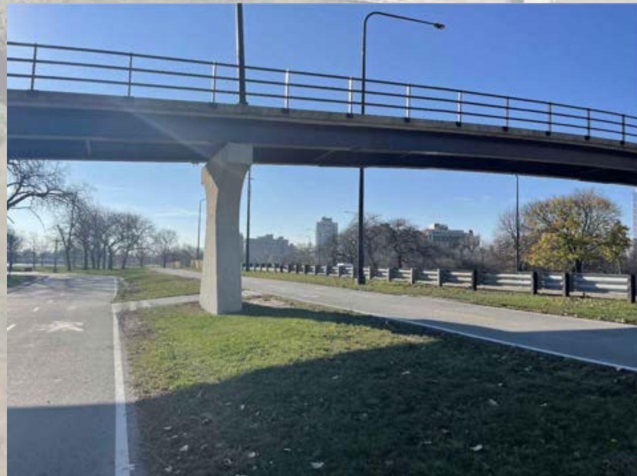
PHOTO A EXISTING 51ST STREET PEDESTRIAN BRIDGE ABOVE PEDESTRIAN AND BICYCLE LAKEFRONT TRAILS
