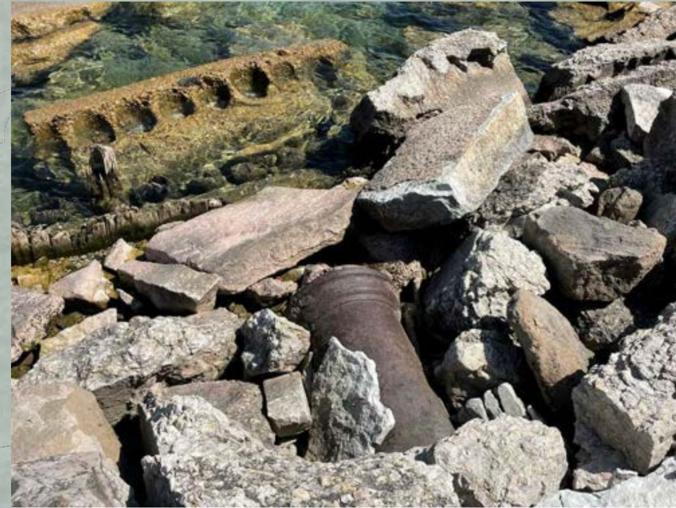
PHOTO B EXISTING 18-INCH CITY OF CHICAGO SEWER OUTFALL THROUGH DETERIORATED REVETMENT
