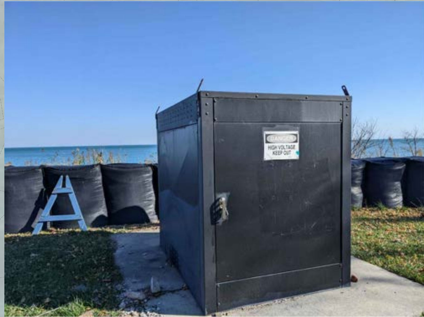
PHOTO A EXISTING ELECTRICAL TRANSFORMER PROTECTED BY BIRD'S EYE SAND TRAPBAGS
