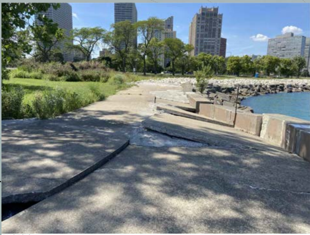
PHOTO C EXISTING UNDERMINED CONCRETE SLABS AND DETERIORATED REVETMENT
